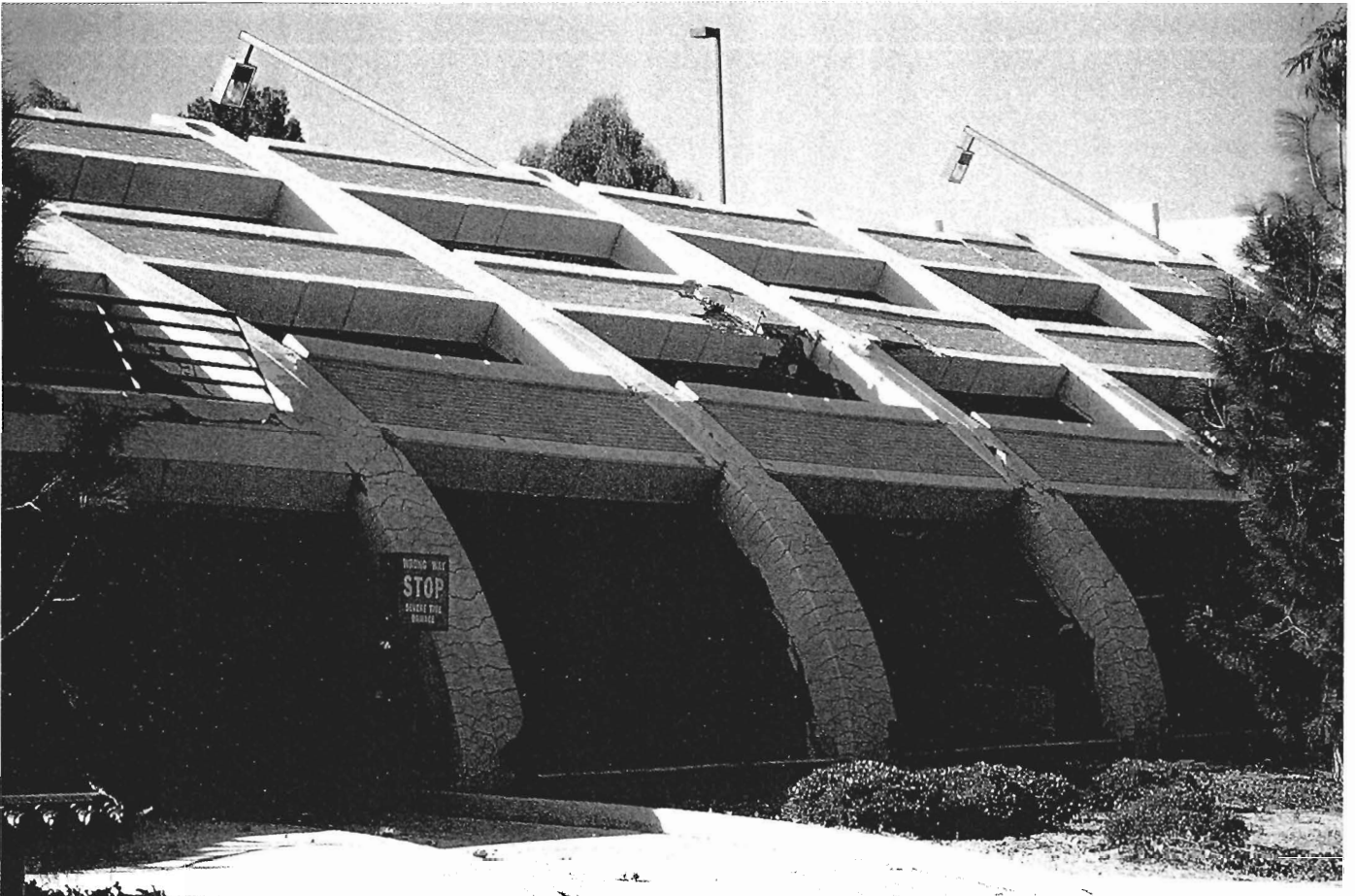
Above: Collapse of a parking structure at California State University, Northridge. The elements of the precast structure were inadequately tied together, giving insufficient lateral load resistance. The columns have sustained enormous deformations without shearing.
